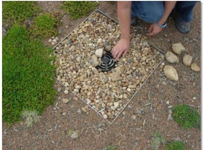
Photograph GR-5. Metal edging separates substrate from rock that surrounds the roof drain. It also serves to facilitate regular maintenance by limiting plant and root growth near the drain.
