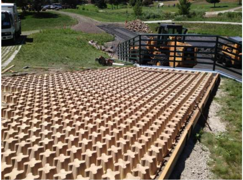
Photograph PPS-16. Forms for concrete grid for reinforced grass pavement to access pond outlet structure.
