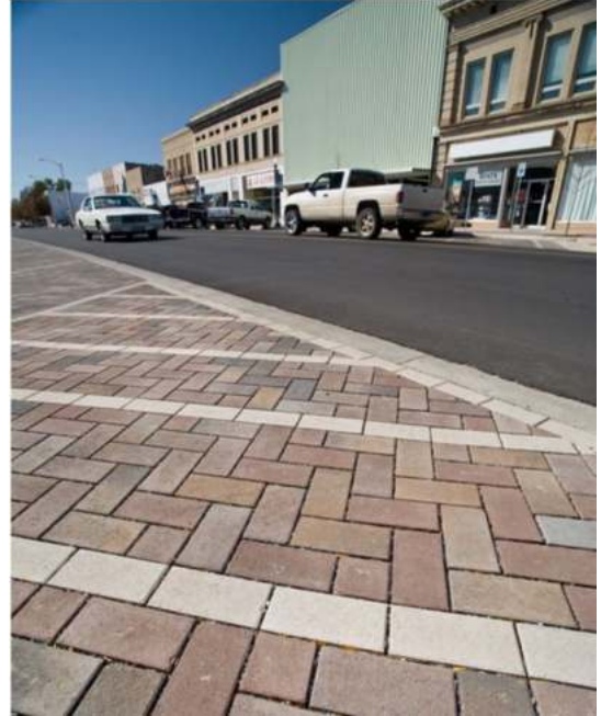
Photograph PPS-3. PICP in downtown Ft. Morgan, CO. Note soldier course of light-colored pavers where PICP meets conventional pavement. Photo: SEH and the City of Ft. Morgan.
