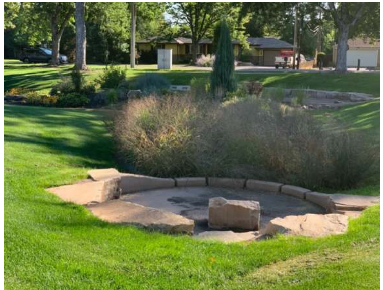
Photograph 4-16. Morse Park forebay provides energy dissipation with placement of a boulder, and the dense vegetation helps encourage sediment to stay in the forebay. This is an easily accessible area to remove sediment and trash, and it provides even distribution of flow to the SCM.
