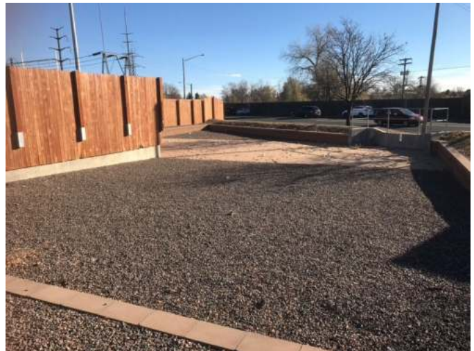
Photograph SF-3. Sand filter with incorporation of minor event flood attenuation provides water quality and detention for a substation.
