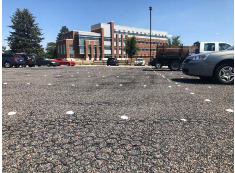
Photograph PPS-5. PGP with grid for containment of surface material to minimize potential for rutting. Photo: True Grid.
