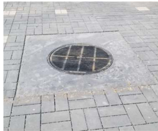
Photograph PPS-15. Concrete collar helps avoid small-cut pavers around edges of inset features and can be colored to match surrounding pavers. Photo: Creative Civil.
