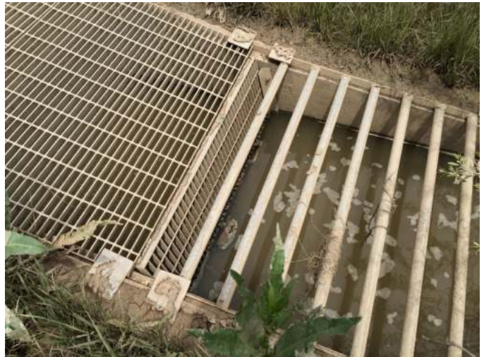
Photograph EDB-6. In this outlet, runoff flows through safety grating (5-inch clear bars) to separate floating debris before continuing through standard bar grating that extends to the bottom of the micropool. The grating extending down into the micropool can be raked through the gap in coarse safety grate to clear debris.
