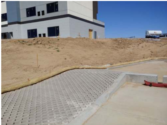
Photograph PPS-18. Concrete cellular paving grid for RGP provides maintenance access to the forebay. Photo: Creative Civil.
