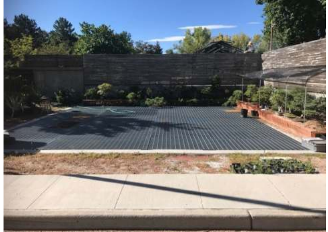
Photograph SF-2. Underground sand filter at Denver Botanic Gardens has a grated top, which enables inspection and maintenance.
