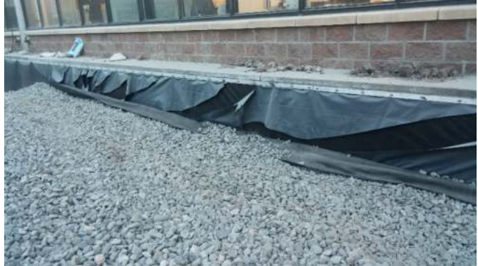
Photograph 4-5. Liner tear after aggregate placement (even with slack provided). To avoid this problem, delay attaching the liner to the perimeter barrier with a batten bar until after placing aggregate by temporarily anchoring the liner
