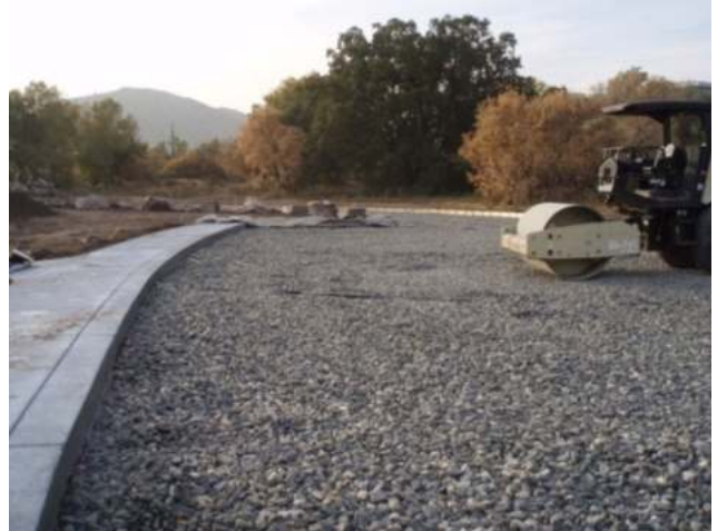
Photograph PPS-9. The reservoir layer of a permeable pavement provides storage volume for the WQCV. Photo: Muller Engineering and Jefferson County Open Space.
