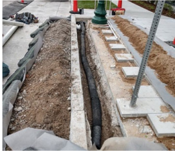
Photograph PPS-7. Perimeter barrier and trench with underdrain to protect street subgrade with adjacent PPS installation. Photo: Beck Group.
