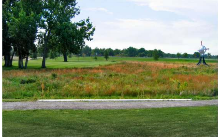
Photograph 4-13. Level spreader at Aurora Sports Park evenly spreads flow to the wetland area downstream.
