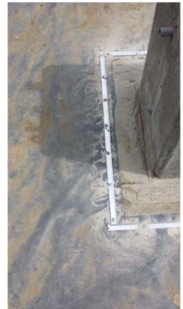
Photograph PPS-11. Geomembrane attachment to horizontal footing for light pole. Photo: Creative Civil.
