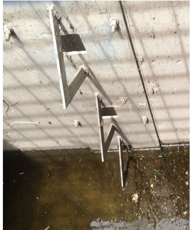
Photograph EDB-4. Where orifices are large enough to omit well screen, trash deflectors can be used in combination with standard bar grating to reduce the likelihood that debris will plug one or more orifice.
