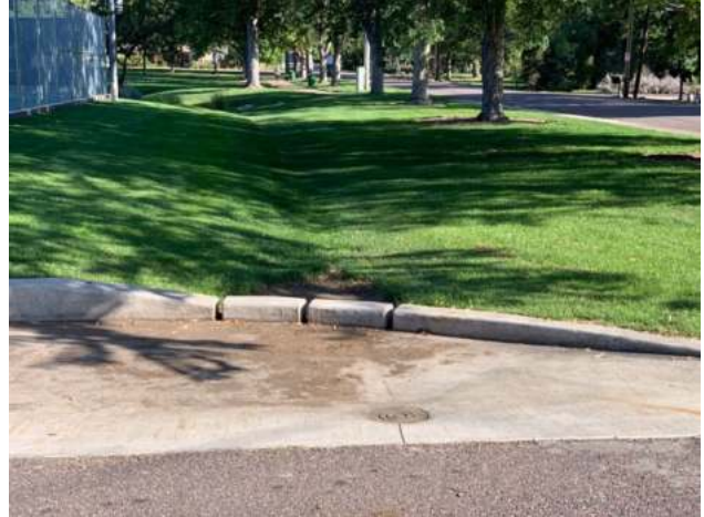
Photograph RPA-10. Sediment forebay at the entrance to a grass swale leading to an EDB concentrates maintenance needs at entrance of swale. This is an example of a three-step treatment train: forebay, swale, pond.
