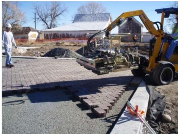
Photograph PPS-20. Mechanical placement in larger areas can reduce the unit cost of the pavement. Photo: Muller Engineering Company and Jefferson County Open Space.
