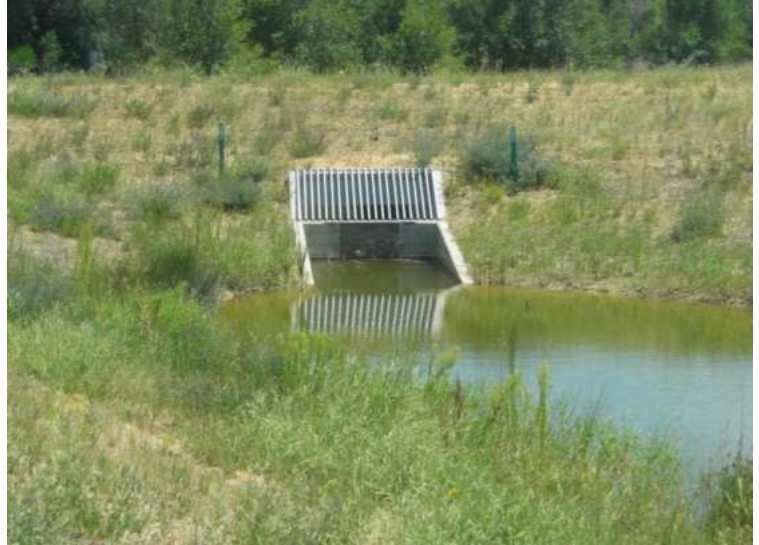
Photograph 4-18. Although each site is different, most sedimentation SCMs have similar outlet structures. Each structure should include a partially submerged orifice plate with a screen (or grate) protecting the orifice plate from clogging, and an overflow weir for flows exceeding the WQCV or EURV when full spectrum detention is used.
