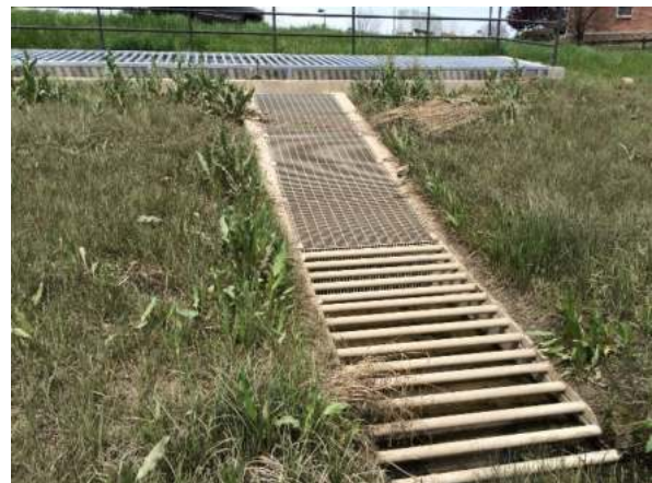
Photograph EDB-3. Outlet structure with coarse safety grating covering the micropool in the foreground, standard bar grating flush with the top of parallel concrete wingwalls and extending down through the micropool, and coarse safety grating covering the 100-year drop box in the background.
