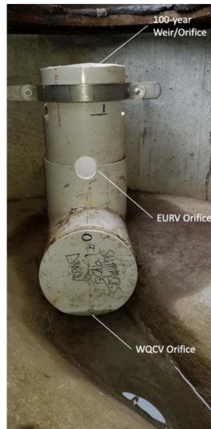
Photograph PPS-13. FSD outlet for PICP system. WQCV orifice is drilled in front of cap at bottom. EURV is controlled by the circular orifice midway up the riser. The 100-year event is released via rectangular orifices on the sides of the riser just below the band. The open top of the riser provides an emergency overflow. Photo: Creative Civil.
